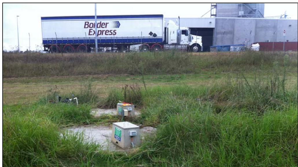
Figure 1: Allied Mills STP (01.03.2011). Aeration tanks shown. Septic and balance tanks hidden in long grass on right of picture. Mill in background.
